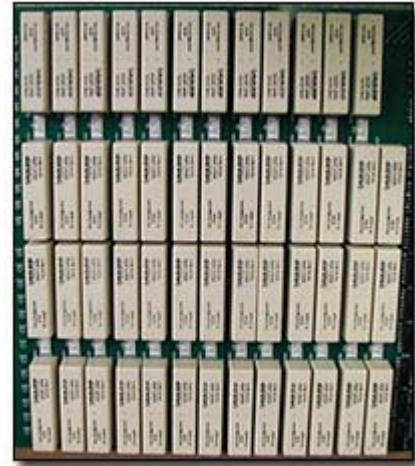
This is the wrong way to do it! Relays are too close and not alternated end-to-end
